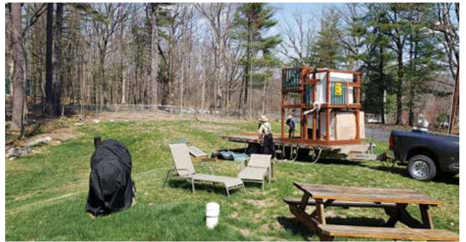
LAYING THE GROUNDWORK: THE SOON-TO-BE-ASSEMBLED PLAY SET ARRIVES IN THE YARD OF HAMASPIK OF ORANGE COUNTY'S SUMMIT BRIDERHEIM IRA GROUP HOME
